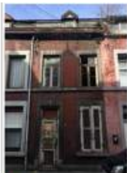
A. State of ruin, safety danger
