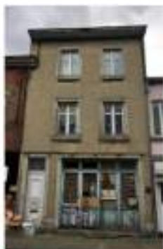
B. Need of heavy renovation
